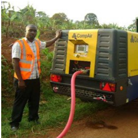
Air compressor for fiber blowing
